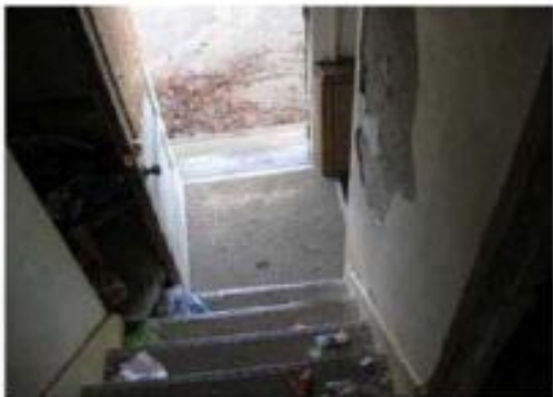
Bid missing handrail
