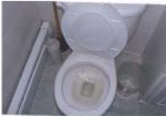
Winterization - Toilet Before
