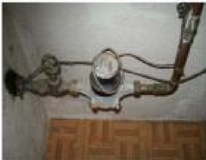
WATER METER BEFORE
