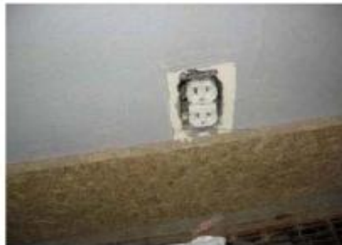
Bid missing outlet cover
