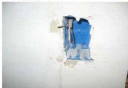
Bid uncapped wires
